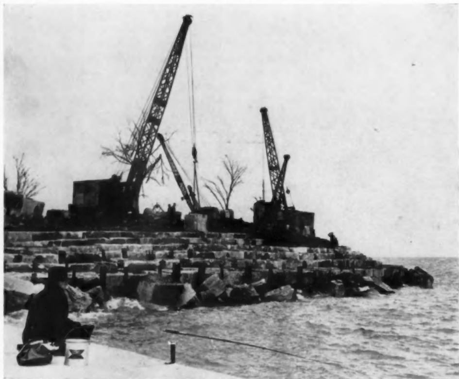
Crane setting limestone blocks into sea-wall at Diversey Parkway and Lake Michigan in Chicago. Blocks are often set in tiers, as in the picture, or they are piled at random.— Chicago Tribune photo.
